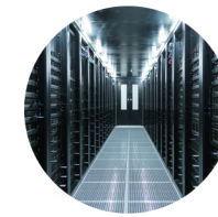
通信系统 Communication system
