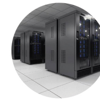
紧急备用电源 Emergency backup power supply
