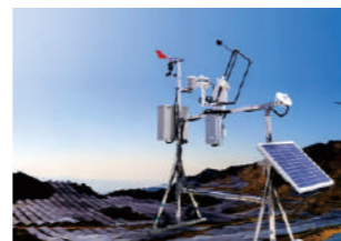
Photovoltaic environmental monitoring instrument
