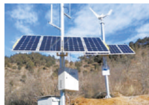
Base station/cell tower
